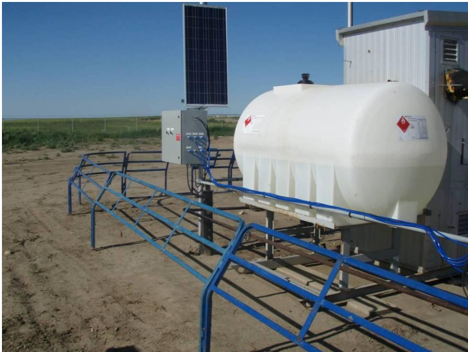
Pic 1. Airwell Pump Solar Powered Control and SCADA System
