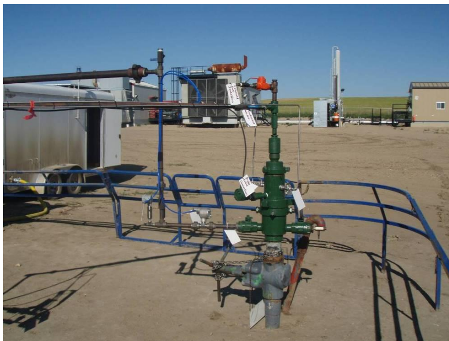
Pic 2. Coiled Tubing Well Head
