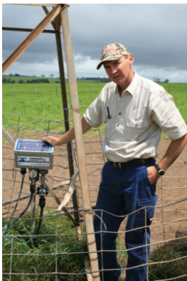
Testing the water: David Bunge checks one of his two Airwell pumps
