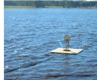
One of Nine Airwell dam pumps at Jigsaw Farms
